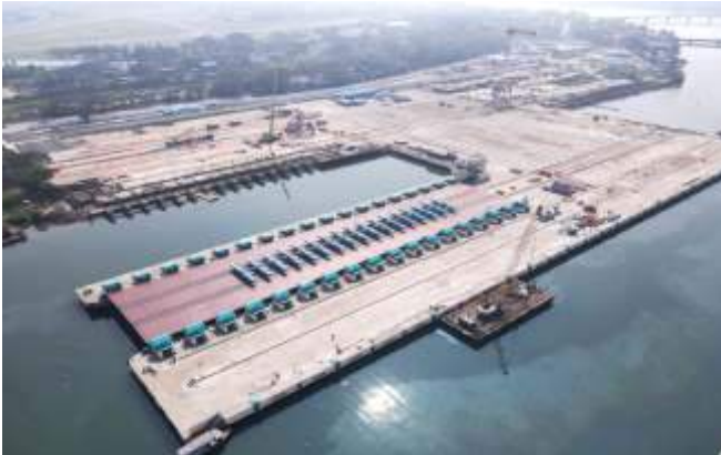
M/s. Syncrolift, Norway, delivered ship lift platform having size 130*27 meter. and 2000 T approx., at ISRF site of CSL on 18 th September, 2023
